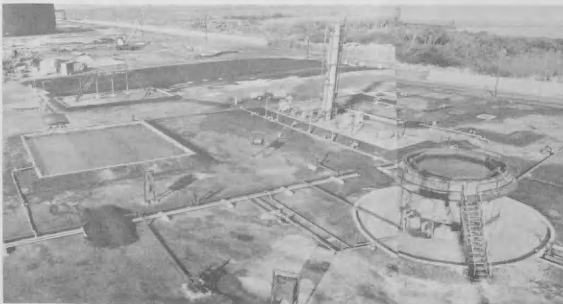
Partial view of improved fire training facilities. Vista parcial di facilidadnan mehora pa sinja paga candela.
